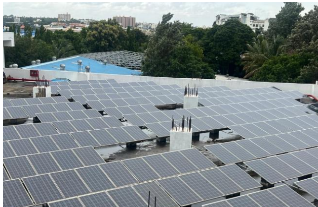
Solar Panel Projects continue with three more plants going live in FY24
